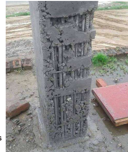
Placing issues (honeycomb)
